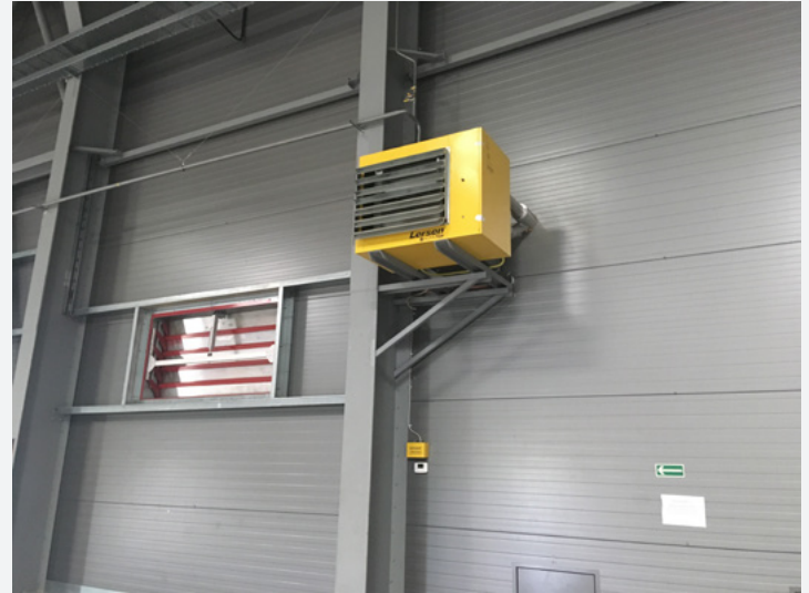
GAS HEATING SYSTEM
